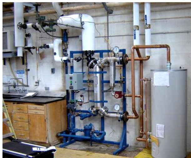
Duplex 65 gpm Domestic on 125 psi steam
